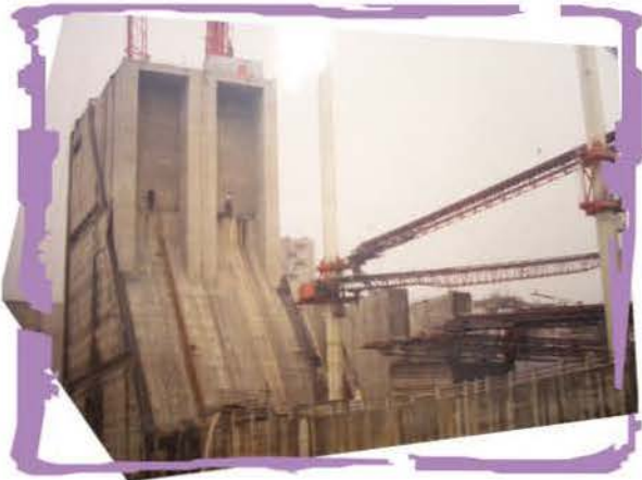
The dams of TGP are 180 metre in height
